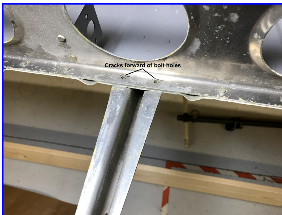
View of center flap hinge. Cracks were found on the outer flap hinge.
